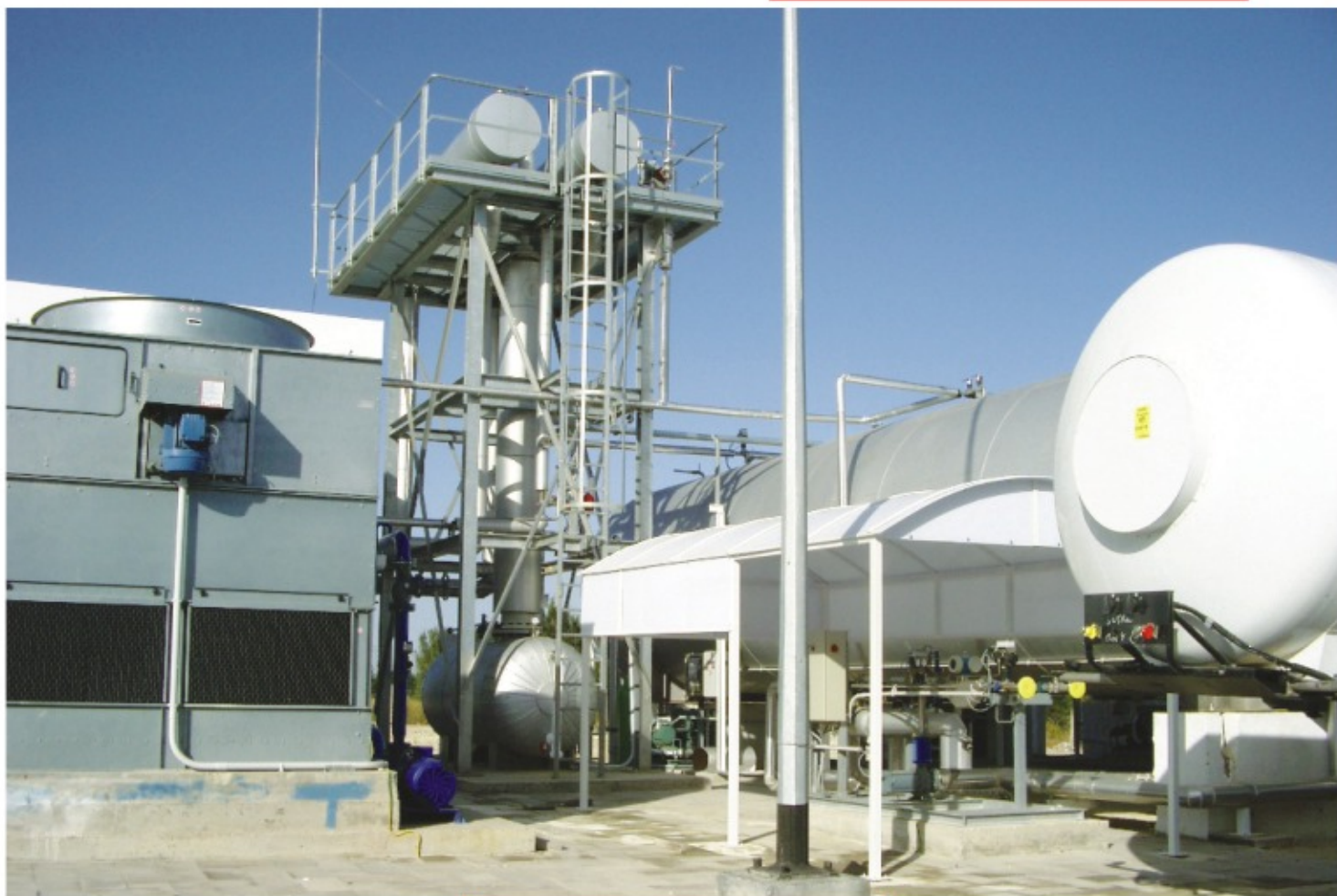
CO 2 Stripping System 3 tons per hour
